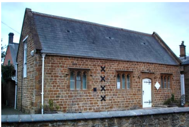
Adderbury Library was built in 1818 as the parish Sunday School. It is closed all day Monday and Wednesday and open for a total of only 18.5 hours per week. If it were closed the nearest library “hub” would be Banbury, to which the adult return bus fare is £5.50.
